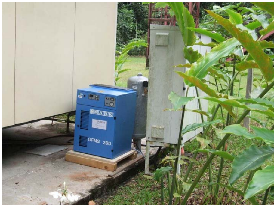
Figure 1: New compressor an Danum Valley
